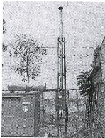
DG Set and stack
